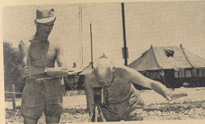
"IF YOU WORK UNTIL 2200 HRS EVERY DAY YOU CAN HAVE SUNDAY OFF". Pte PADDY O'NEILL (Left) and Sgt John Joe Murray of IRCON Engineers don't seem unduly perturbed as they prepare another site for building.
